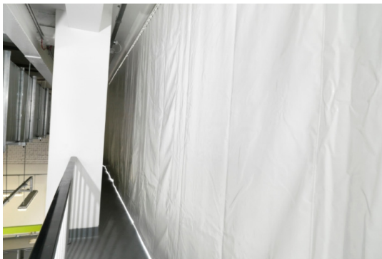
Laser Safety Curtain installed in Imperial College, London
