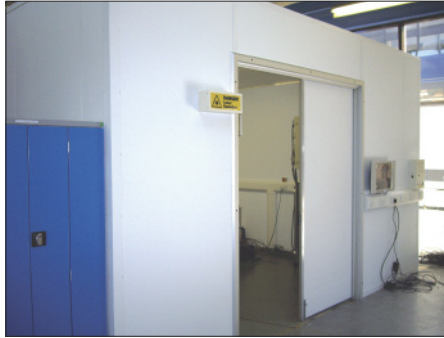
Laser enclosure with interlock system and CCTV
